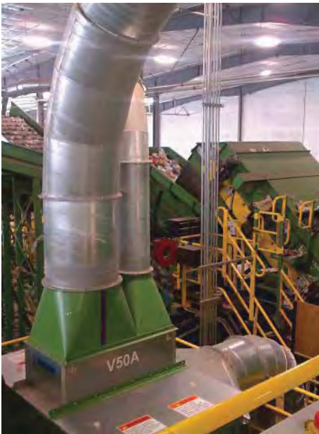
State of the art plastic vacuum system.
