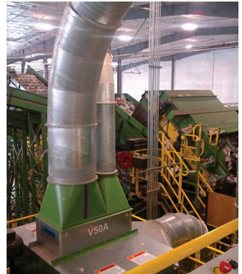
State of the art plastic vacuum system.
